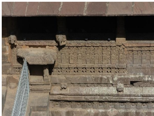
Figure 5 Vedibandha present at Chand Baori, probably the remnants of the earlier temple.
